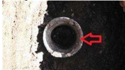
Missing effluent filter
