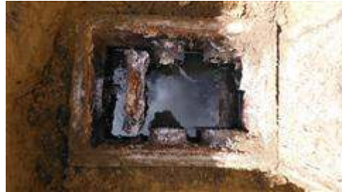
D-Box. Note deteriorated baffle
