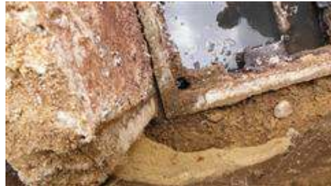
Small crack in D-Box
