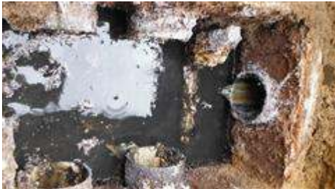
Deteriorated baffle in D-Box
